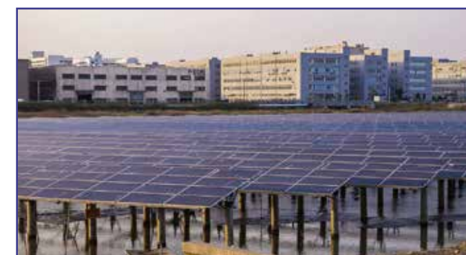
100MW Ningde City, Fujian Province
